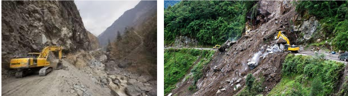
Figure 5.2.4 Landslides due to road construction
